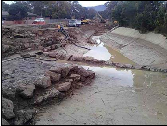
Widening of Brushy Creek, upstream of Bellara Drive, during Stage One works
